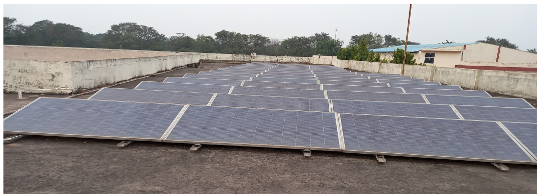
A View of Solar Power Plant
